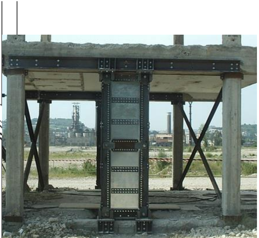
Seismic upgrading of existing RC buildings by means of metal shear panels: design models and full-scale tests – F. Mazzolani – U Naples
